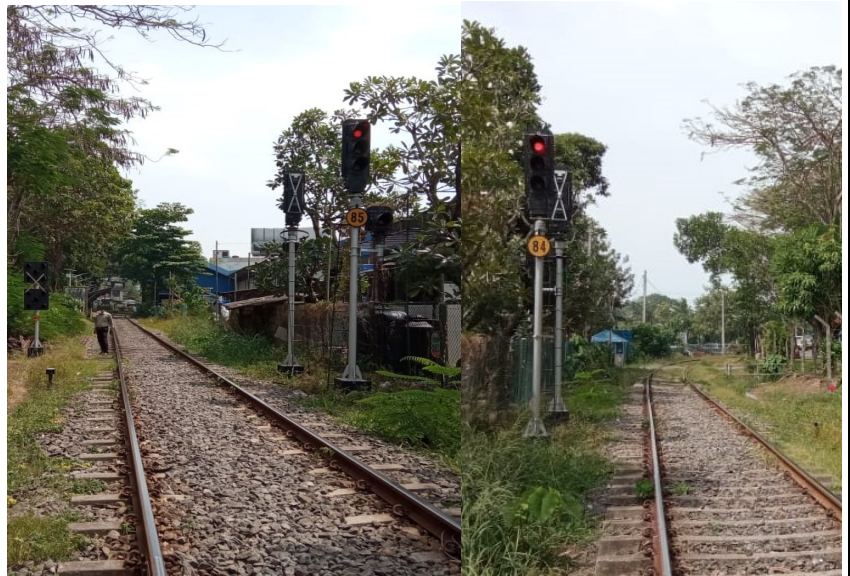
MAG Approach Signal and Nawinna Automatic Block Signal
