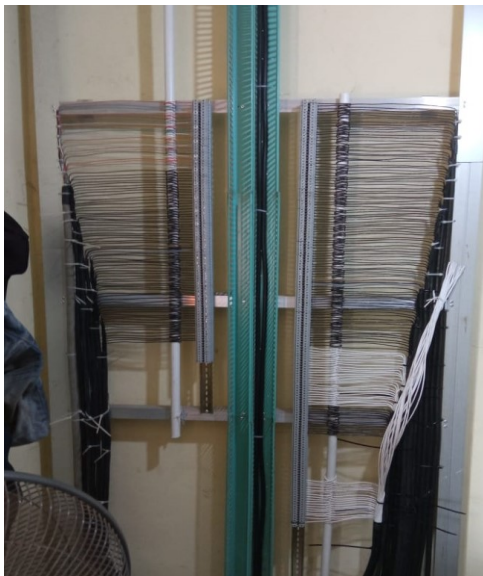
Cable Termination Inside B Type Relay House
